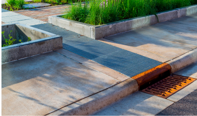
A storm inlet designed as a catch basin sump in LaCrosse, WI.
